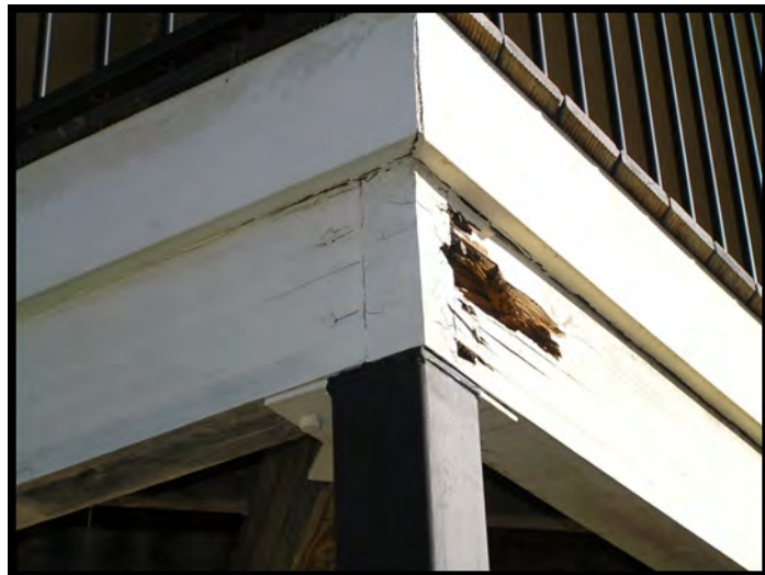
Decay of untreated, non-durable Glulam beams in full weather exposure (Brisbane).
