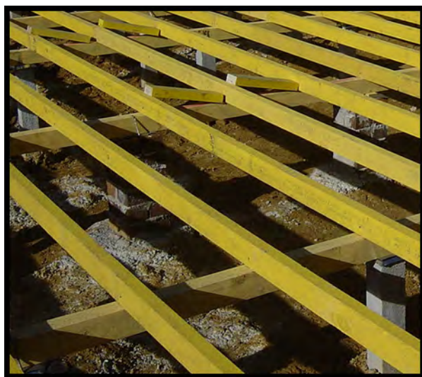
LVL sub-floor frame treated H2 for termite resistance. (Courtesy CHH WoodProducts Australia)
