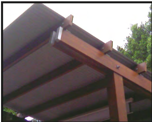
Exposed Glulam beams protected from weather using metal end capping (Breakfast Creek Pub, Brisbane).
