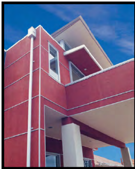
Stained exterior plywood cladding.
